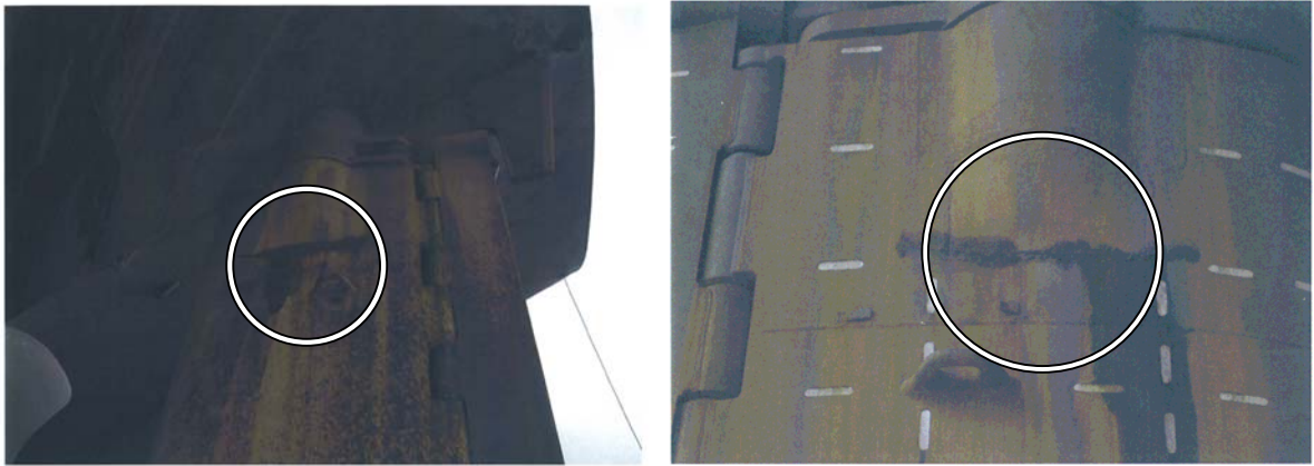
Typical cracks below the conical coupling
