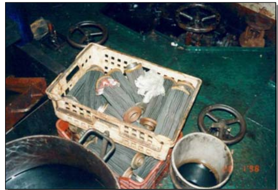
Improper storage/handling of filter elements
